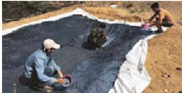
ThaiBev's employees construct tilapia fish pond (claying waterproofing clothes) for a student lunch program for students at Baan Srikeereerak School.
